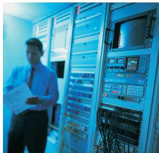
Servers, data storage and network equipment
