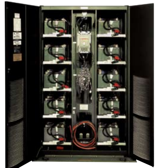
IBC-L with doors opened
